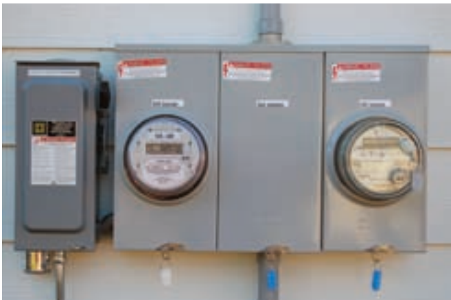
L to R: The solar array's AC disconnect, PV production meter, and utility meter.
